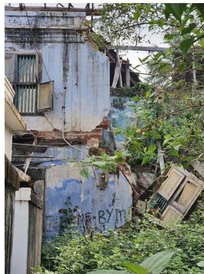
Fig.10.Dilapidated Tharavad (Source: author)
